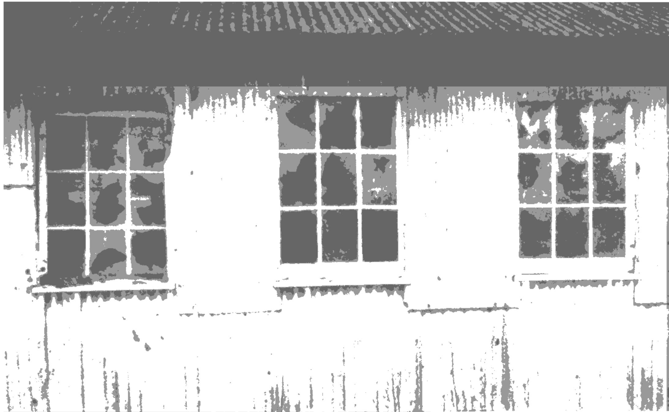
Sutherland's: From the back and inside, the kind of conditions that made the workers want to leave. This is where the hides are worked. It is dark, smelly, and manifestly unsafe.
